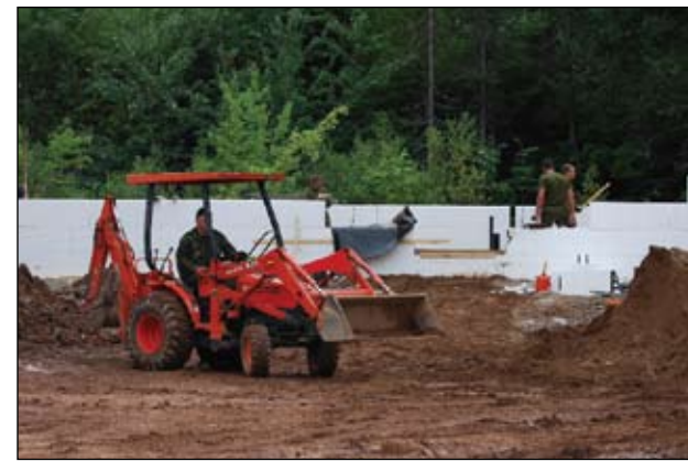
Local military at work on the new Oromocto and Area SPCA Photo: Oromocto and Area SPCA
